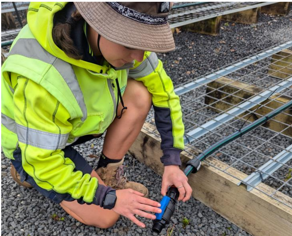
New nursery irrigation system
