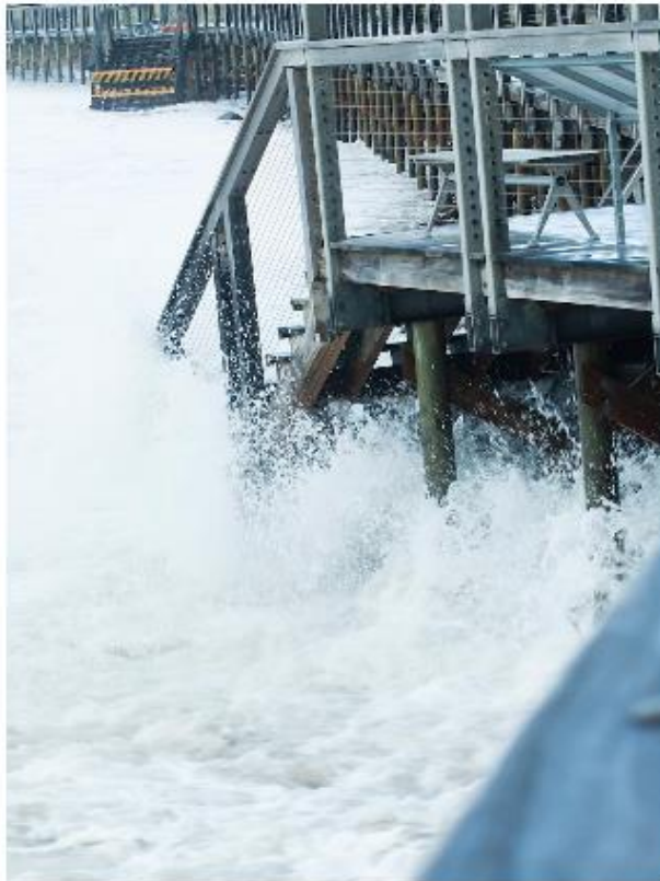
Burnie's prized West Beach walkway was not exempt from damage, with one access point closed for repair. (ABC Northern Tasmania: Rick Eaves)
