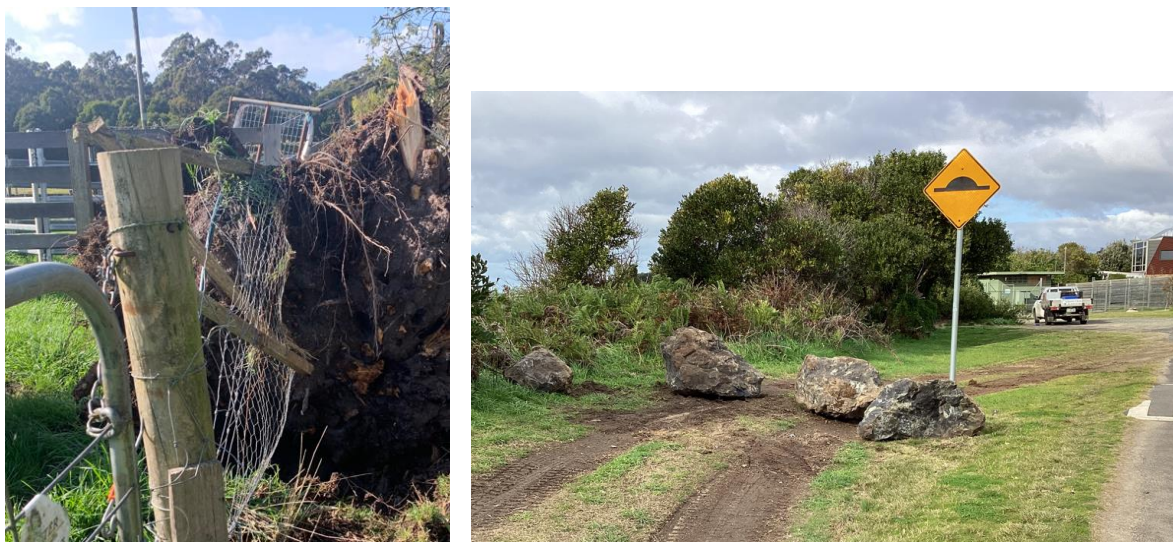
Figures 10 & 11 - Removal of tree uprooted on Pages Rd and installation of barrier rocks at Tennis Crt, Somerset
