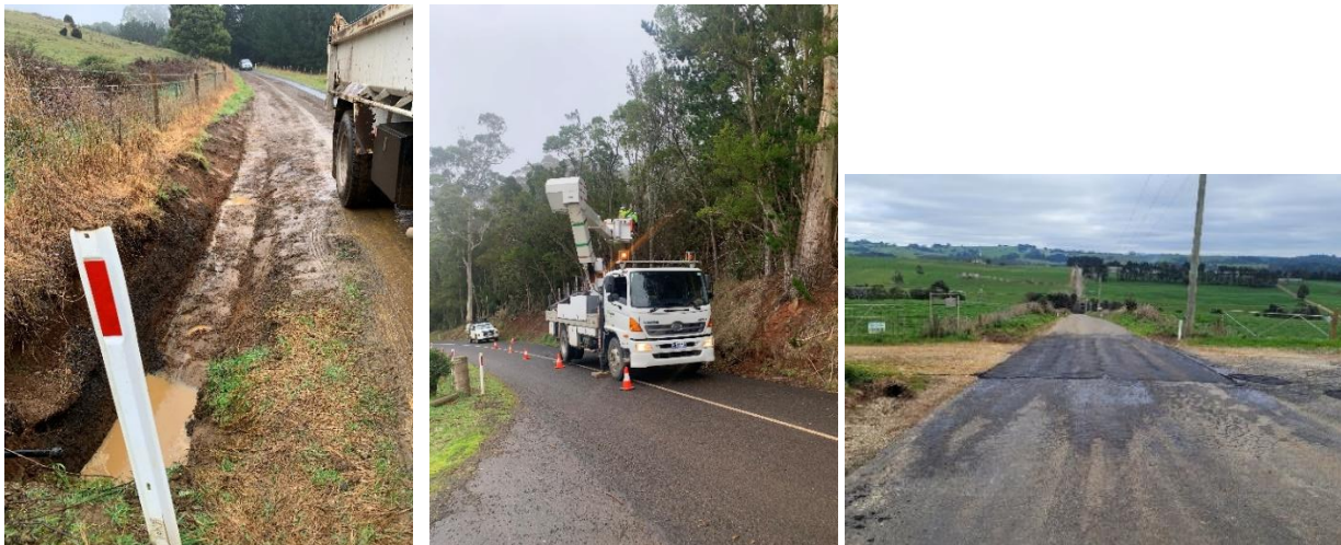
Figures 7, 8 & 9 – Tysons Rd culvert and verge maintenance, typical tree limb hanging that requires attention and section of hot mix replacement over damaged cattle crossing on Nunns Road
