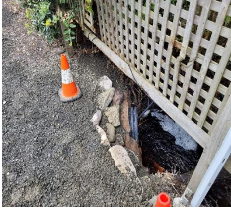
Figures 3 – Culvert maintenance (repaired headwall) on a beach walking track in Sisters Beach
