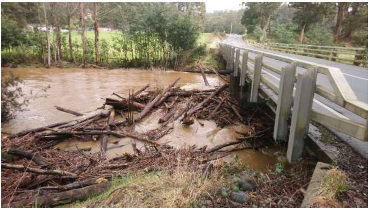
Figure 5 - Logs and other debris build up at the bridge on Pages Road
