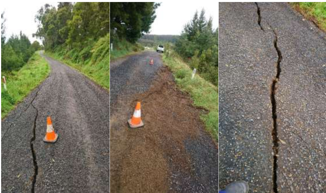
Figure 9, 10 & 11 - Lowries Road slip. This slip continued to move for a week post the initial slip. The road remains restricted to a 5T load limit and the speed reduced. This road is subject to a geotechnical investigation
