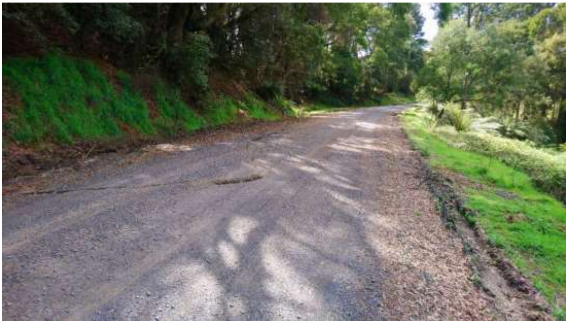
Figure 1 Land/Road slip on South Elliot Road
