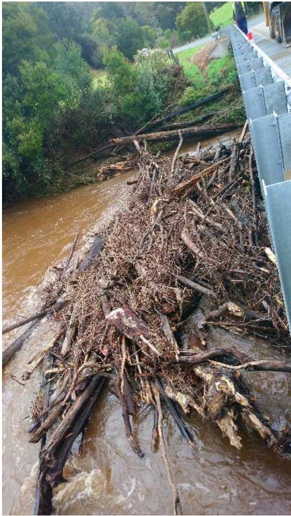
Figure 12 - Debris build up at the bridge on Lapoinya Road
