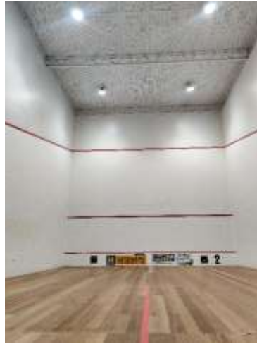
New LED lighting at the Wynyard Squash Centre
