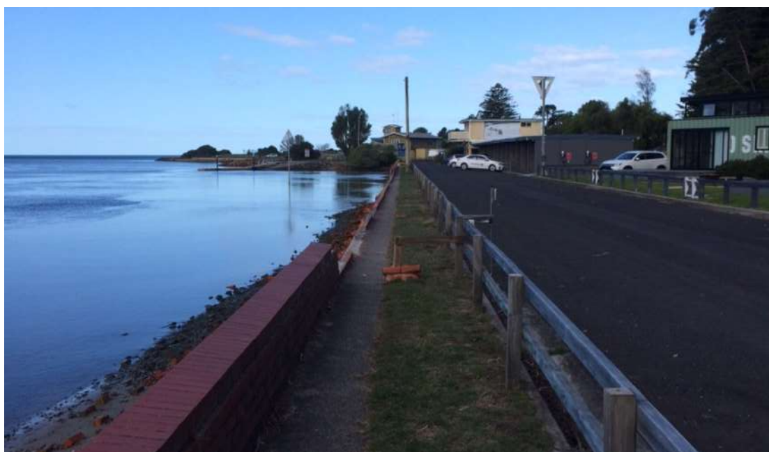
Image 1 - existing concrete footpath and damaged seawall looking east towards the yacht club
