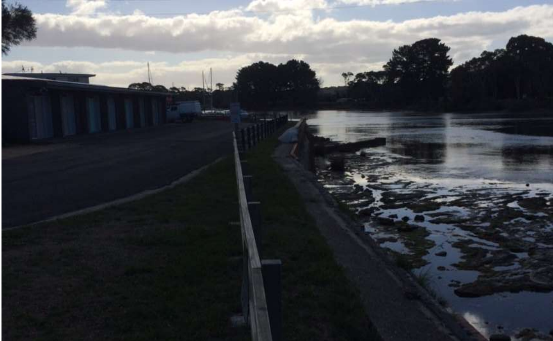
Image 2 - existing concrete footpath and damaged seawall looking north-west towards the wharf
