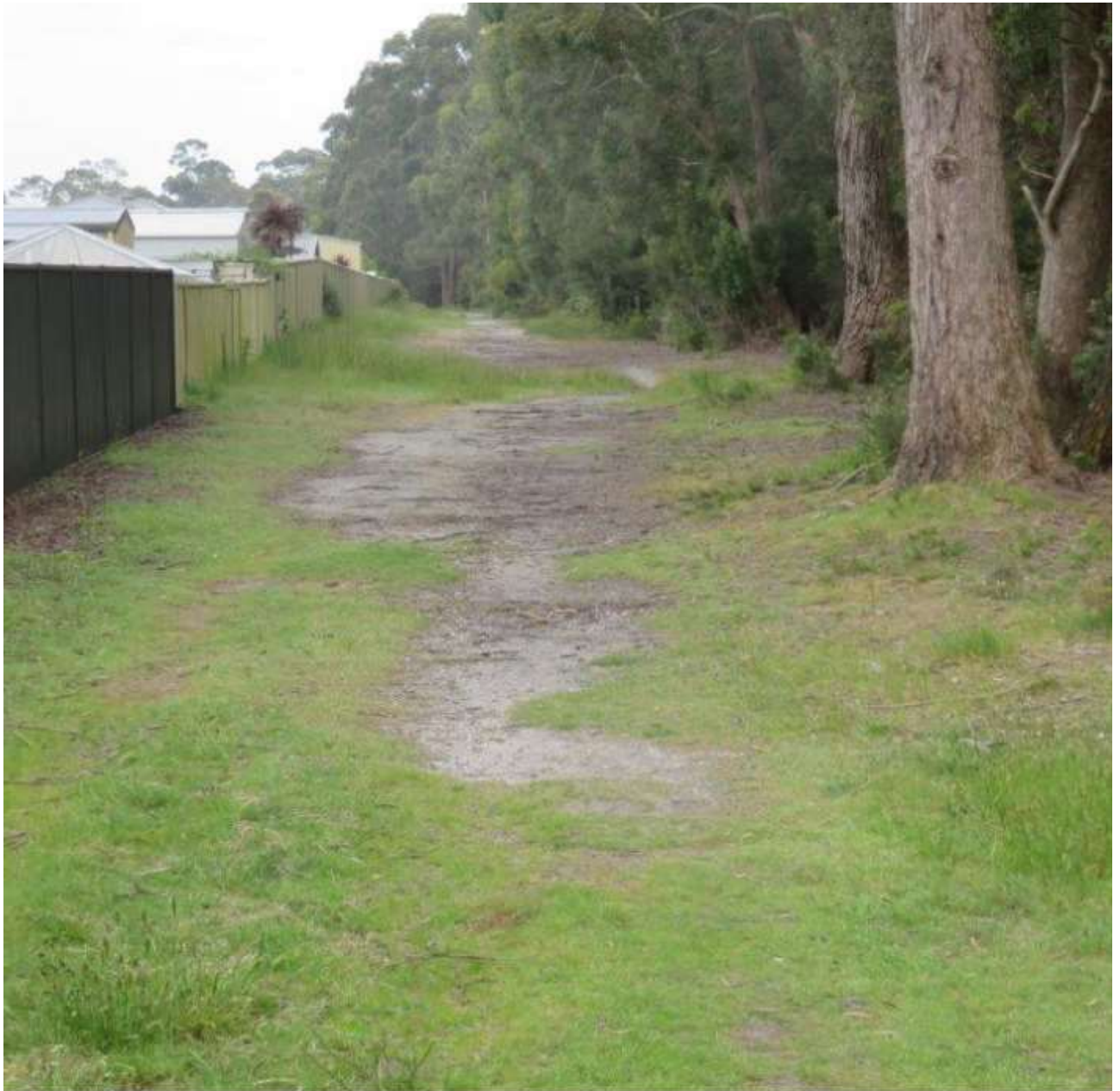
Existing nominal 6m wide fuel break at the rear of Katelyn Drive residential properties
